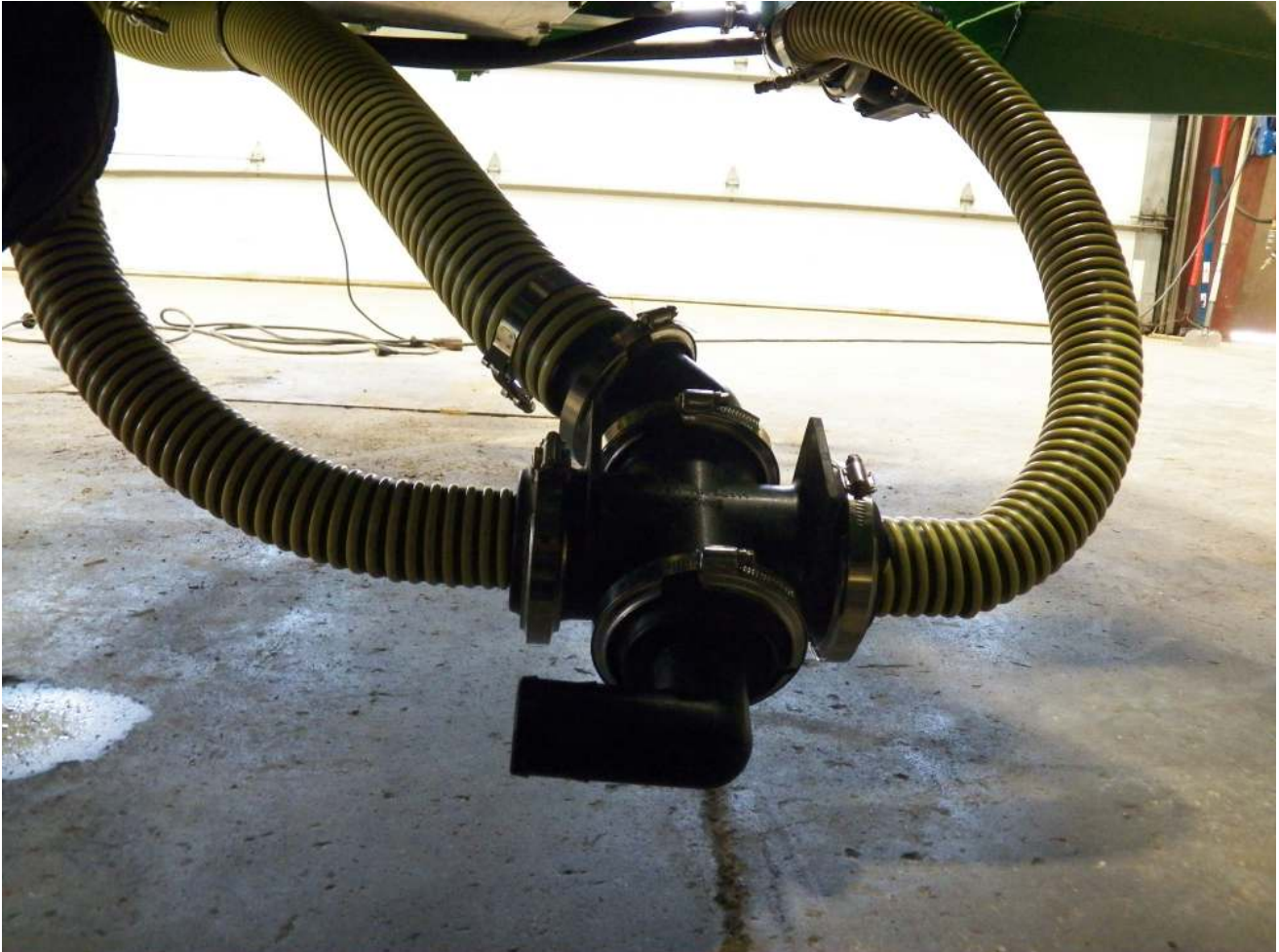
Tank sump and reload plumbing hoses shown hanging for clarity.
