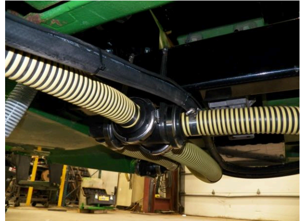
Figure 7: Under-frame plumbing assembly viewed from rear-right.
